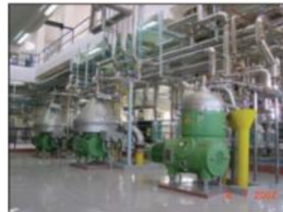
A piping network in an industrial facility.
